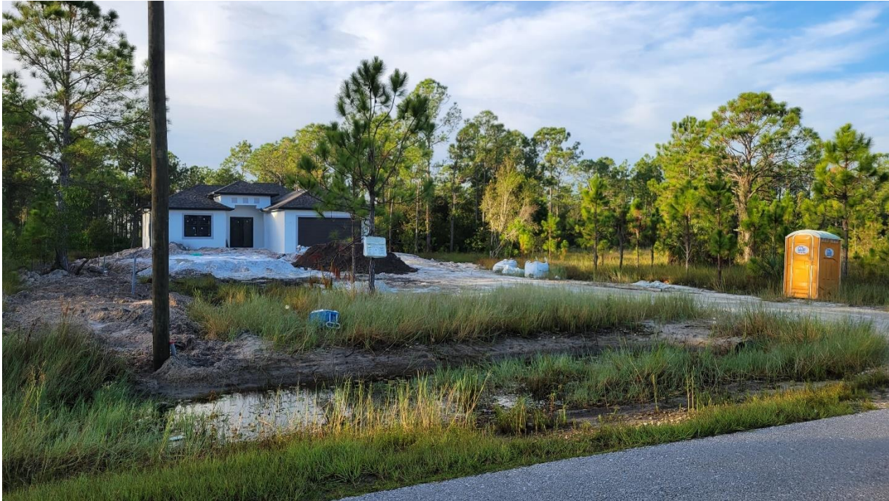
New home being built in pine flatwoods near parcel 20 on 58 th Ave NE
