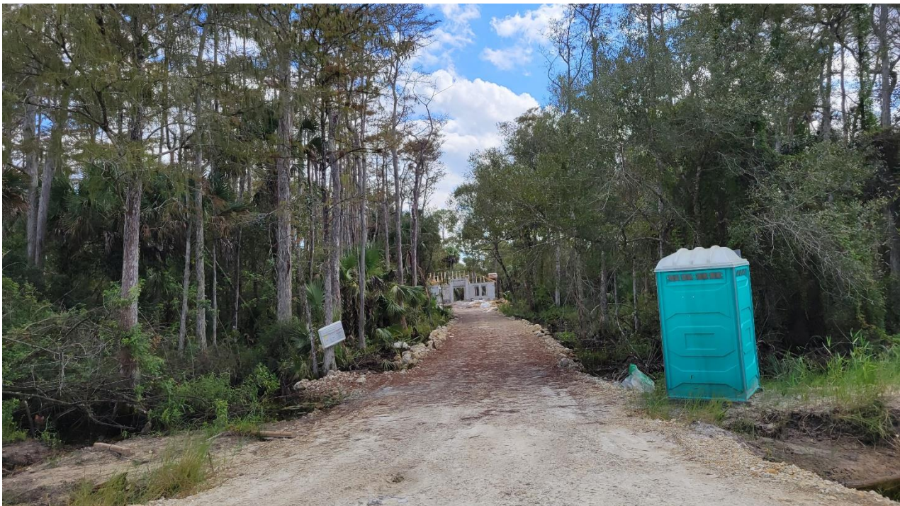
New home being built directly in cypress strand forest near parcel 11 on 64 th Ave NE. New construction displaces water and influences the surrounding hydrology.
